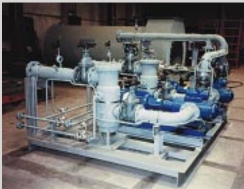
Burner operating valve train for natural gas
