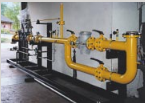
Low pressure-circulation pump station for Bunker C oil
