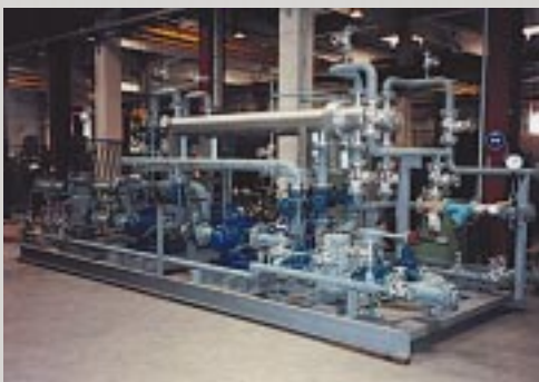
High pressure-filter/pump/preheater-station for Bunker C oil. Heating medium: thermo oil
