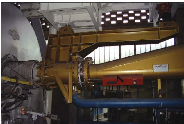
Figure 7. Combined M.A.S kiln burner at W&P cement plant, Austria.
