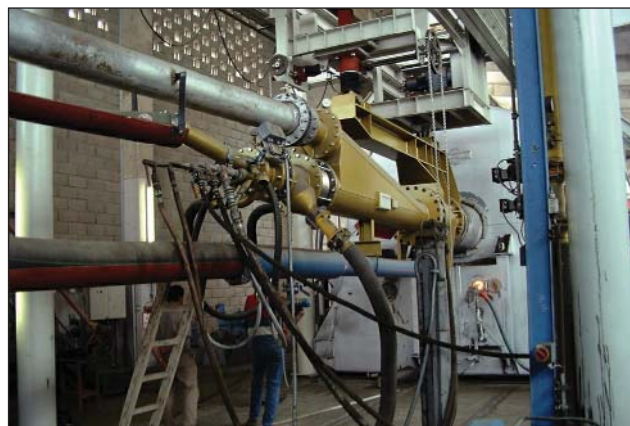
Figure 8. Rear view with fuel connections and new burner trolley.
