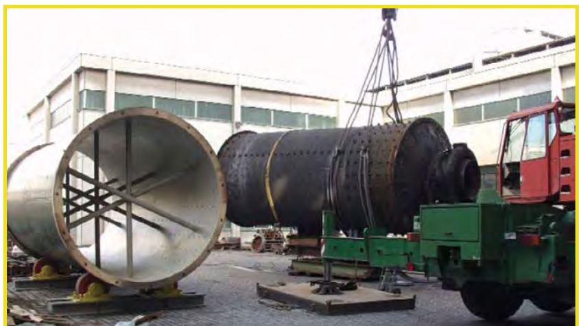
The old mill shell, to the right, was replaced by Teutrine with the new shell (left) supplied by PSP.
