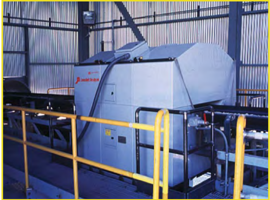
The GammaMetrics CB 1000L on-line PGNA analyser as installed in the quarry.
