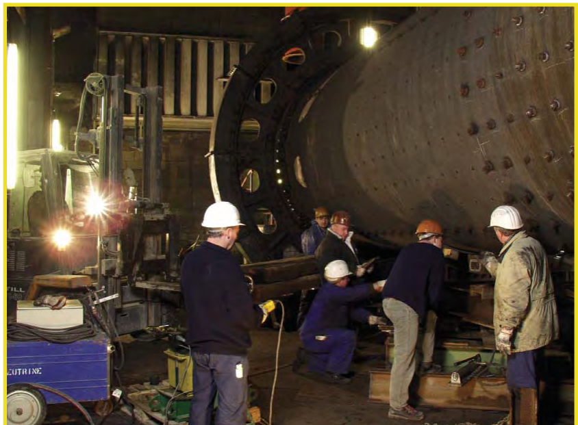
Early stages in the operation to replace the shell of the old coal mill.
