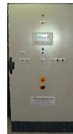
Control System S7
