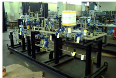
fuel oil valve train for kiln burner
