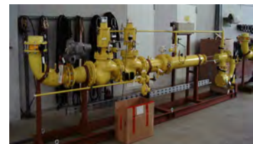
Gas Control Valve Station DN 200
