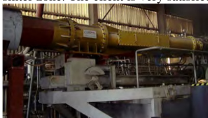
M.A.S. Kiln Burner / Leimen
