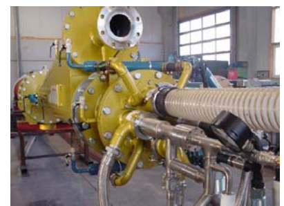
M.A.S. kiln burner for 2 solid waste fuels, coal, HFO fuel oil, and liquid waste fuels. (Holcim)
