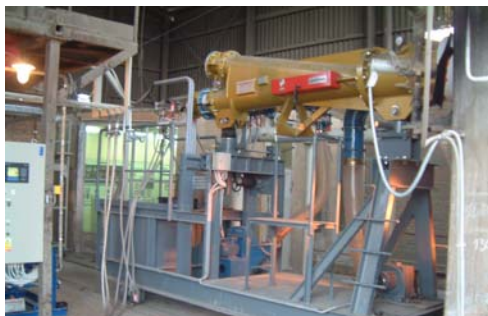
Unitherm installation at Lukavac Cement Plant / Bosnia:
