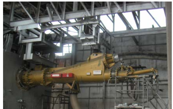
Modern M.A.S. kiln burner installation at Hyundai Dan Yang cement plant designed for 5 different fuels
