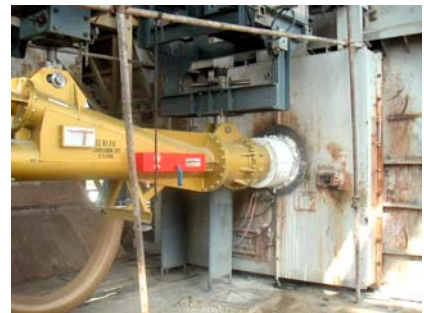
Right: M.A.S kiln burner in operation at Fecto Cement Plant
