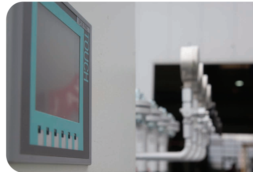
A local operation panel mounted at an oil station
